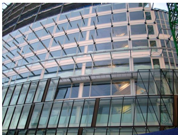
1 Angel Square – showing the inner skin, with the outer skin under construction at the lower part of the
